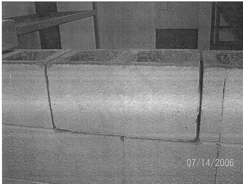
Partitioning walls at this facility have been compromised as a result of settling
