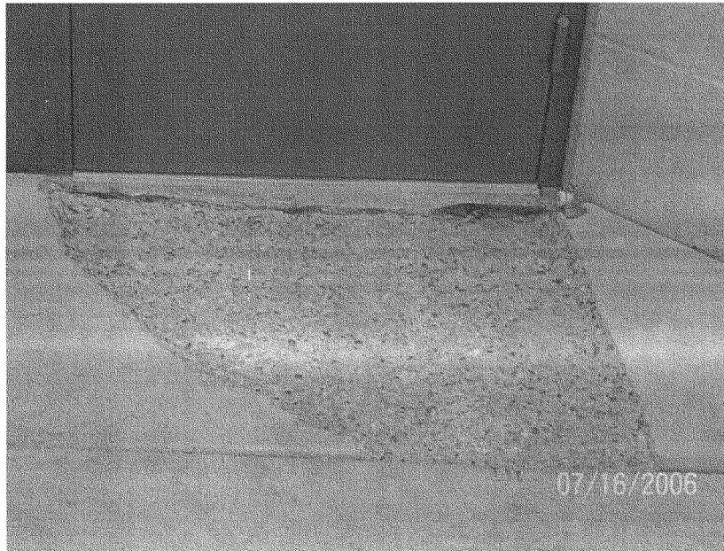
Concrete scraped about 1 inch to allow opening of the exterior door
