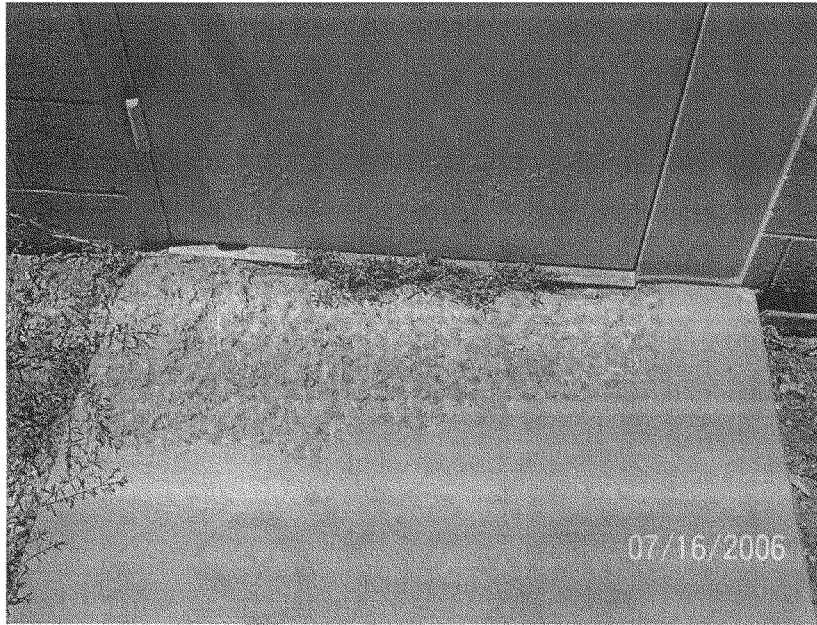
Concrete has to be scraped out to permit opening of the door – which is sinking at a faster rate than the concrete slab outside
