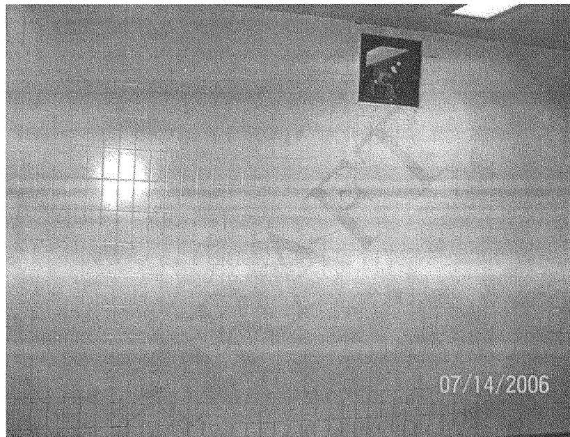
Stress cracks at 45 degree angle indicate settling of the foundation
