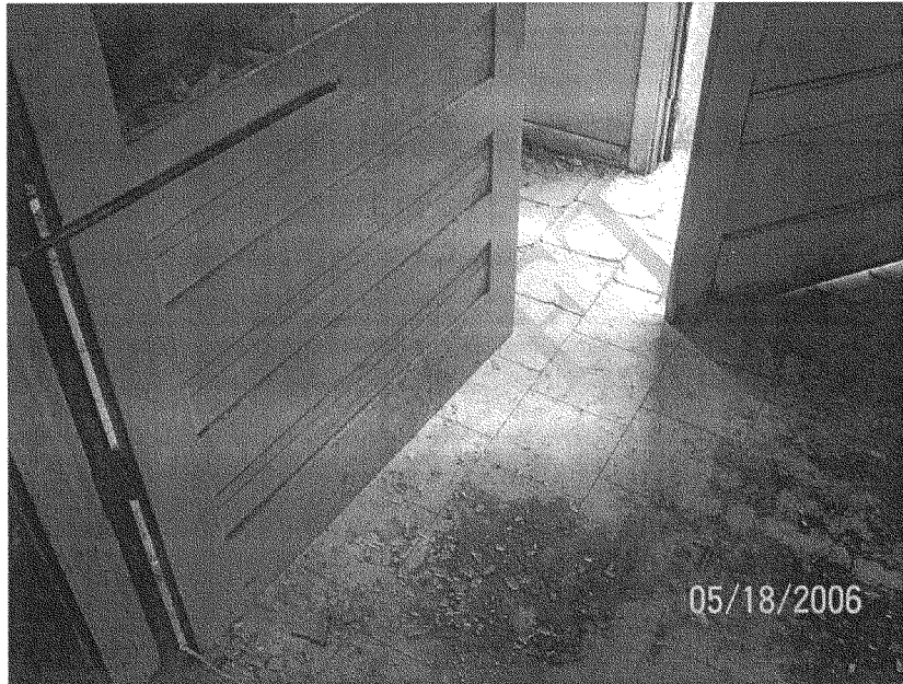
The front door cannot close since the door jamb skewed resulting from the settling foundation.
