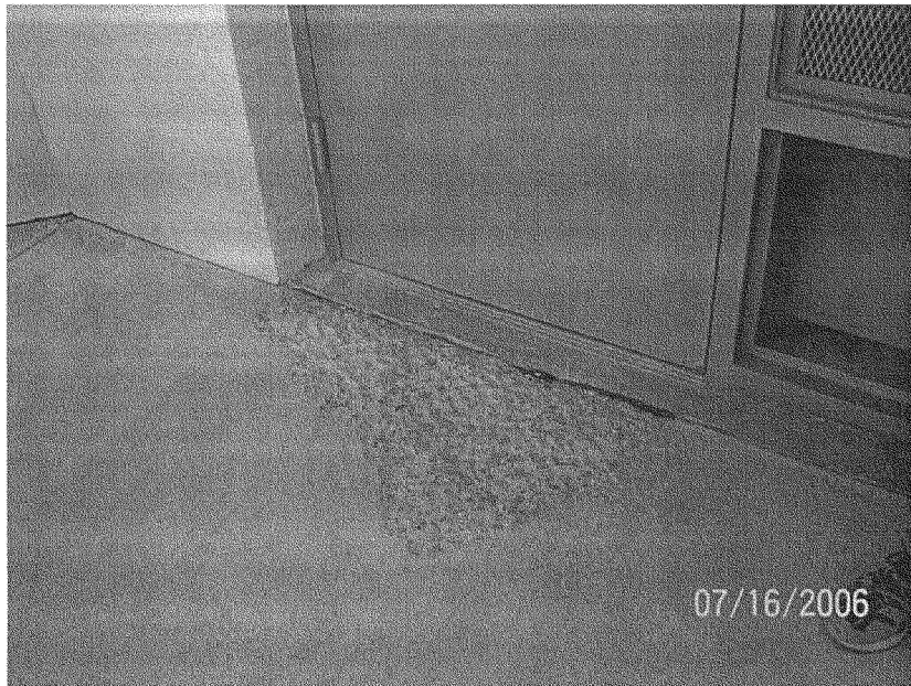
All exterior doors have sunk, some faster than others
