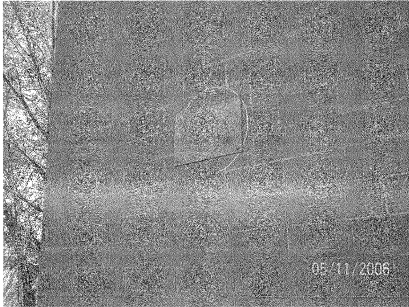
Plywood repair from an escape in the past
