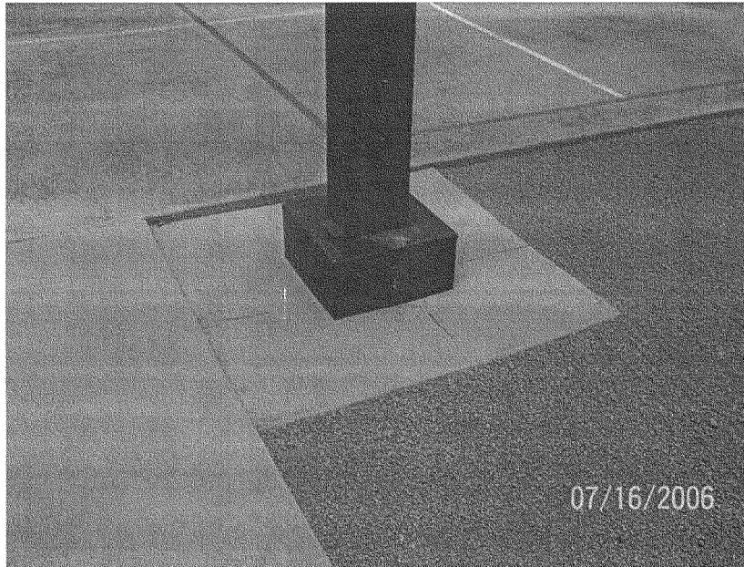
Concrete footing at the base of this outdoor light fixture – that has a vertical weight of about 300 pounds, has settled about 1 inch
