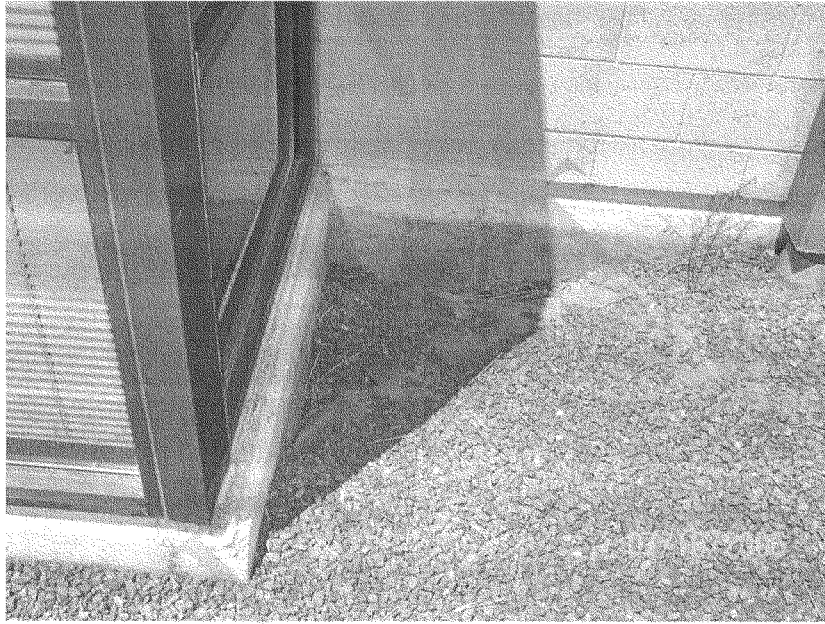
Soil collapse at a corner
