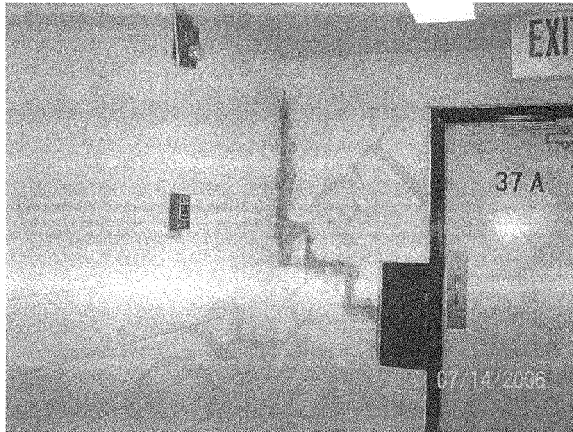
This temporary solution does not resolve the fundamental problem of a settling foundation
