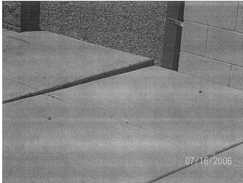
Movement of concrete slab resulting from settling soil
