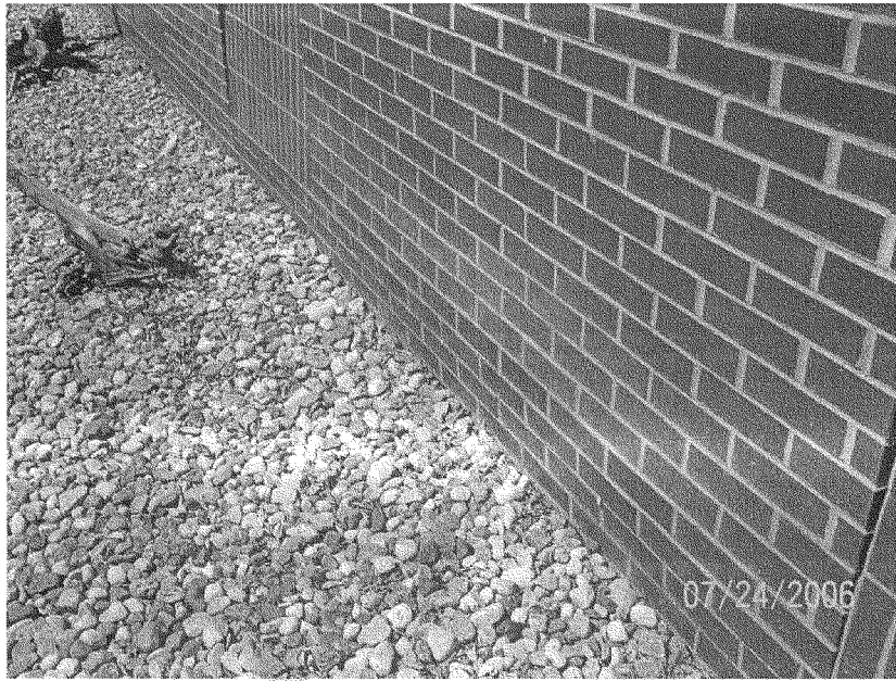
Bulging exterior wall
