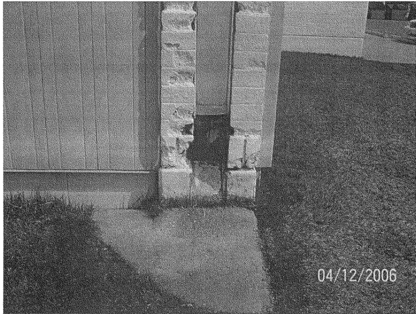
Weathered and crumbled concrete fins
