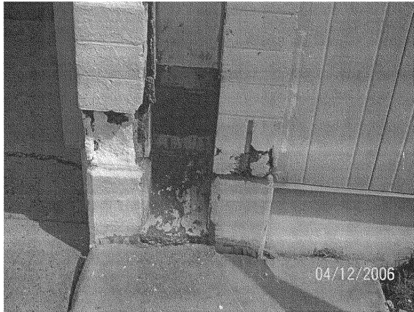
Weathered and crumbled concrete fins
