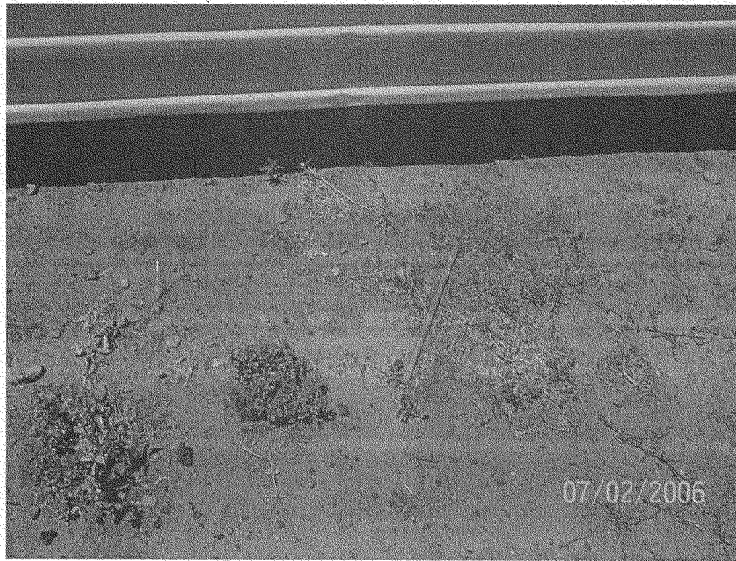
A left-over anchor-bolt dropped when this storage trailer was installed
