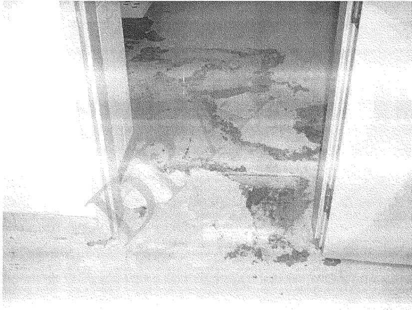
Stains from sewage in the cell, spilled over from the toilet connection at the sink-toilet combination unit
