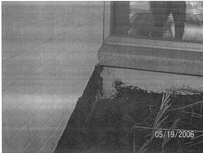
Soil collapsed along the weight bearing edge of the wall
