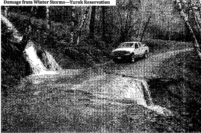
Damage from Winter Storms—Yurok Reservation
